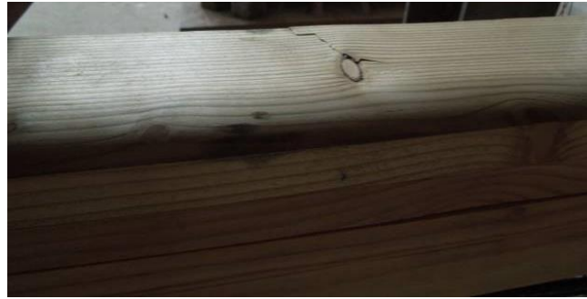
(b) Skew cracks on the surface of the beams
