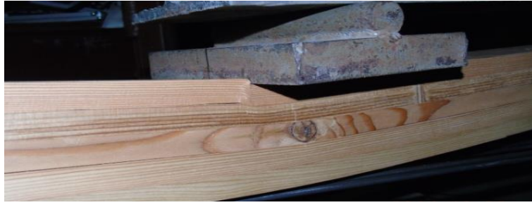
(c) Tension failure of the beam top
