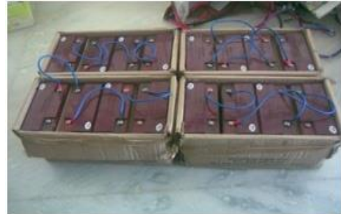
Figure 7. Traction Batteries – 4 x 12V 20Ah
