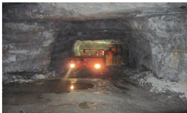
Fig. 9. Drilling by Extra Low Profile Drill Jumbo in Development Face of FW Lode
