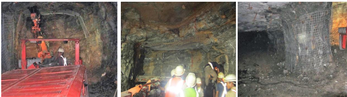
Fig. 10. Fixation of Welded Support Firmly to the Immediate Roof near the Development Face
