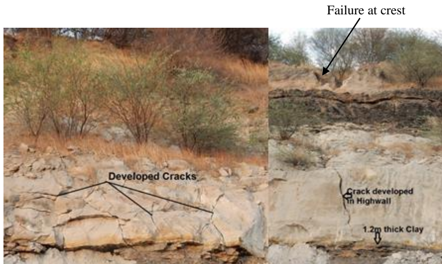
Figure 2.11. The cracks developed due to dipside highwall failure at Medapalli OCP
