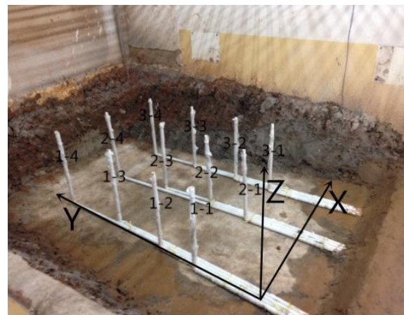
Fig .2. The saturation line piping
